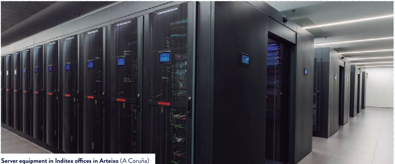
Server equipment in Inditex offices in Arteixo (A Coruña)
